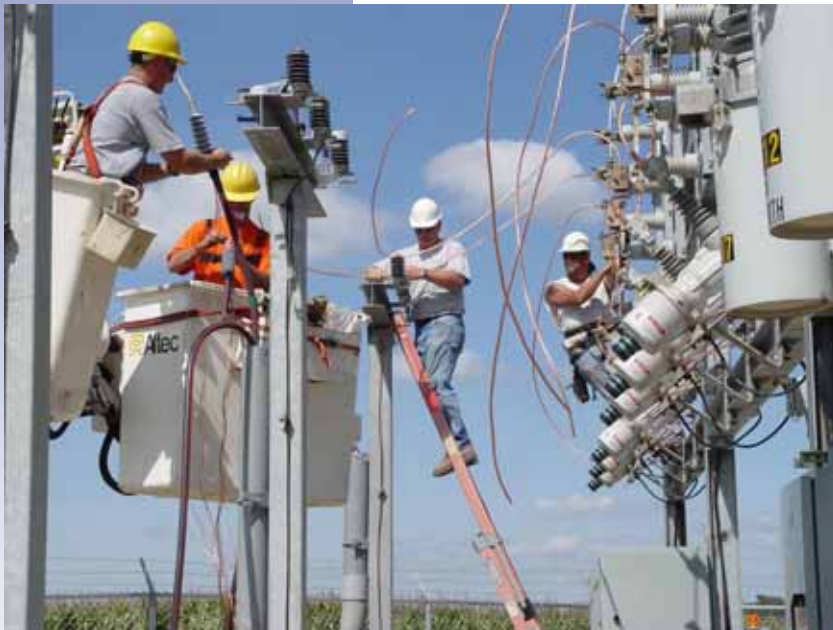
Linemen from North West REC and NIPCO rewire Siouxland Sub as it is doubled in capacity to 10 MVA. From left are Rob Driesen and Phil Elgersma, both of North West REC, and NIPCO’s Steve Harringa and Chad Marcotte.
