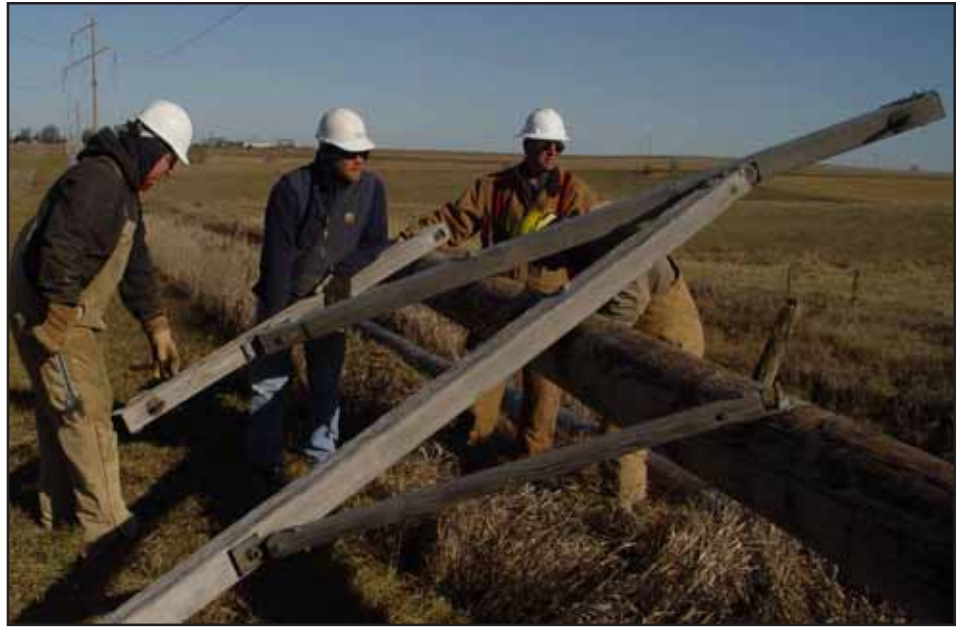
NIPCO crews replace a damaged transmission pole along a dirt road in Cherokee County before winter makes the repair impossible. From left are Steve Harringa, Chad Marcotte, Tom Berkenpas and Roger Armstrong (hidden by the crossarms).
