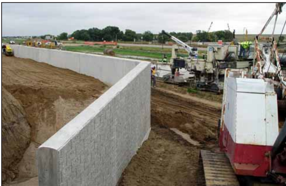
Construction workers pave the southbound lanes of U.S. 75 in NIPCO's front yard in mid-September. Access to NIPCO headquarters has been via a temporary road since April. In late October, construction crews began rebuilding NIPCO's driveway on County Road C-38.
